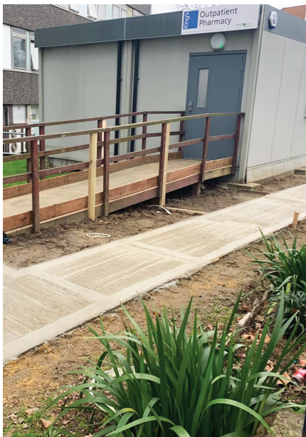
All deliveries redirected to the rear of building to reduce congestion through front entrance.
